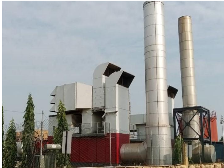
Figure1: Gas Turbine Power Generator GT1(5.2MW) and GT2(5.6MW)
