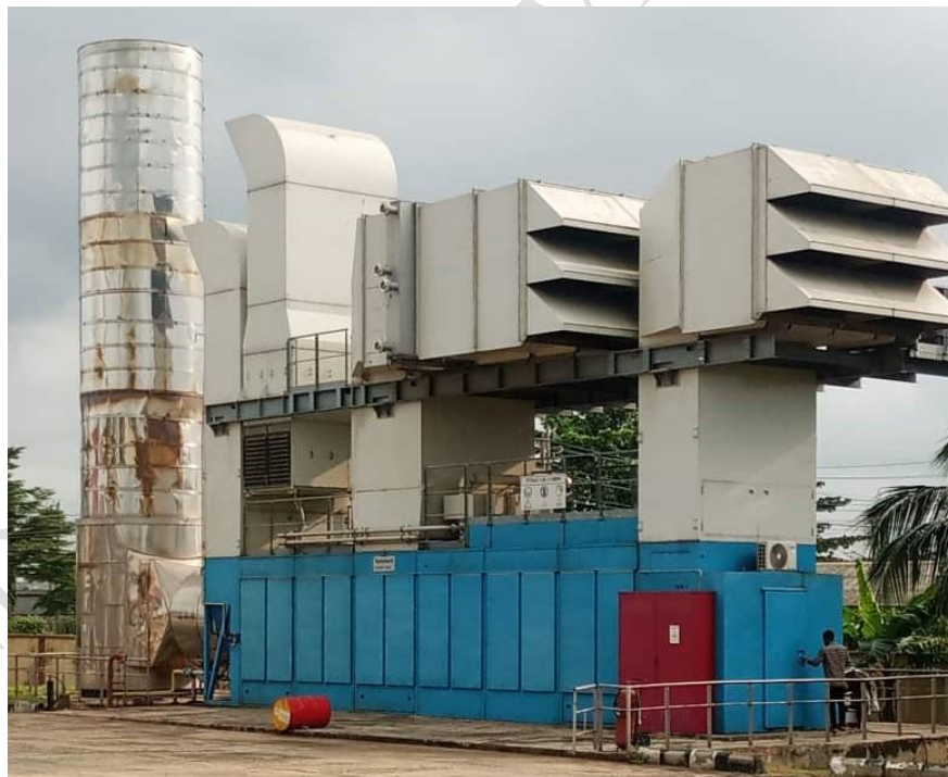
Figure 2: Gas Turbine Power Generators GT3 15MW
