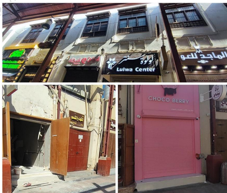
Figure 8: Signage, Façade, and Protection Quality Distortion
