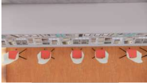
Gambar 4.11 Installation Room Sumber: (Dokumen Pribadi)
